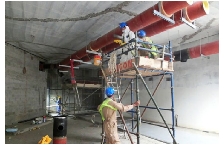
Mechanical, Electrical & Plumbing Services (MEP)
