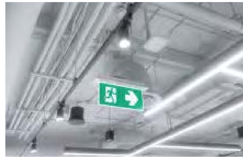
Mechanical, Electrical & Plumbing (MEP)
